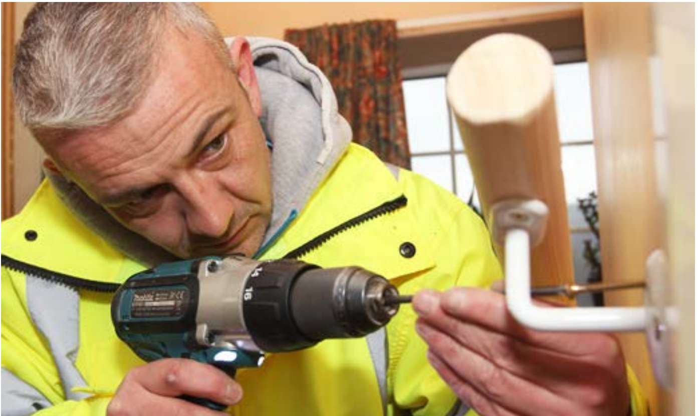
Care & Repair operative installing handrail for a client. Copyright © Care & Repair Cymru.
